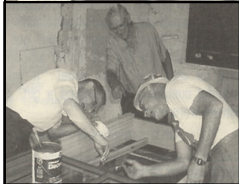
Don Welzenbach explaining restoration plans to visitors (above), Welzenbach painting windows with Richard Muller and Al Tank (below)
